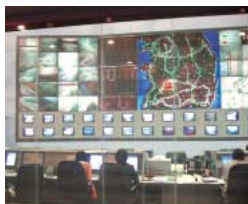
Traffic control center
